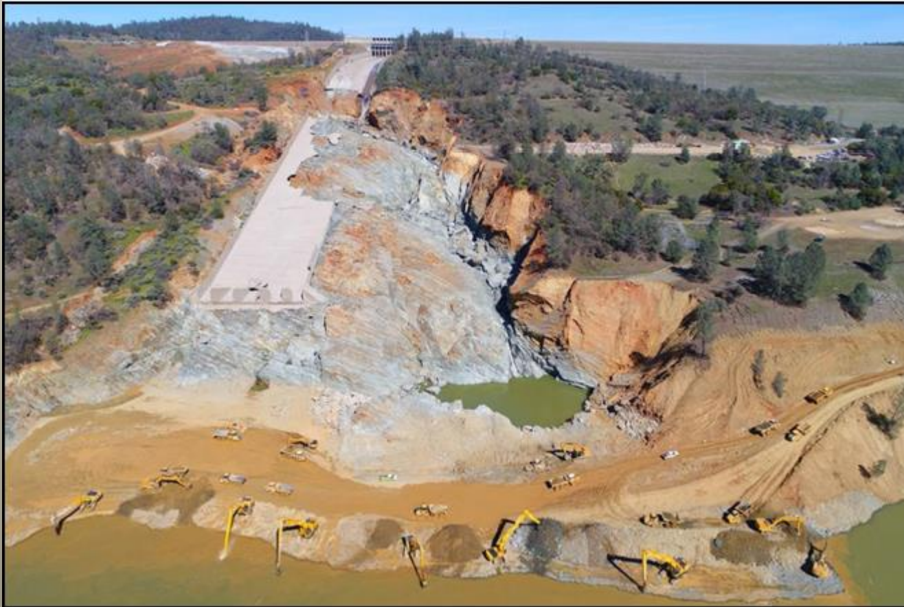
Ultimate damages at the service spillway
