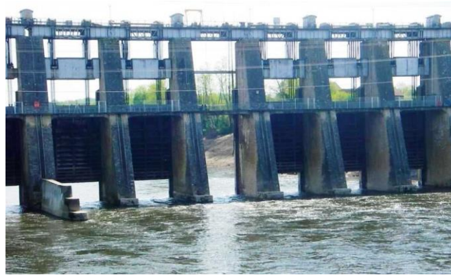
© Photo EDF after #4 Stonley gate failure in 2006
