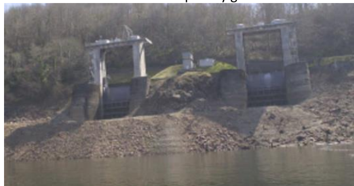
© Photo EDF spillway gates
