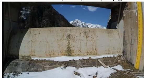
© Photo K. Superd Spillway flap gate
