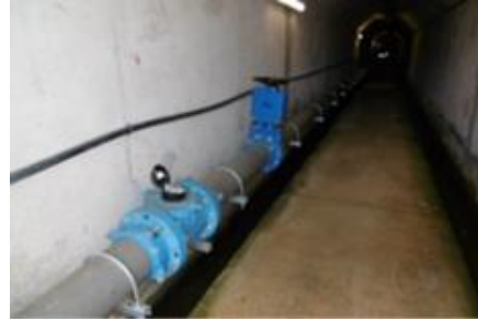
© Photo OEHC Bottom outlet pipe and valve
