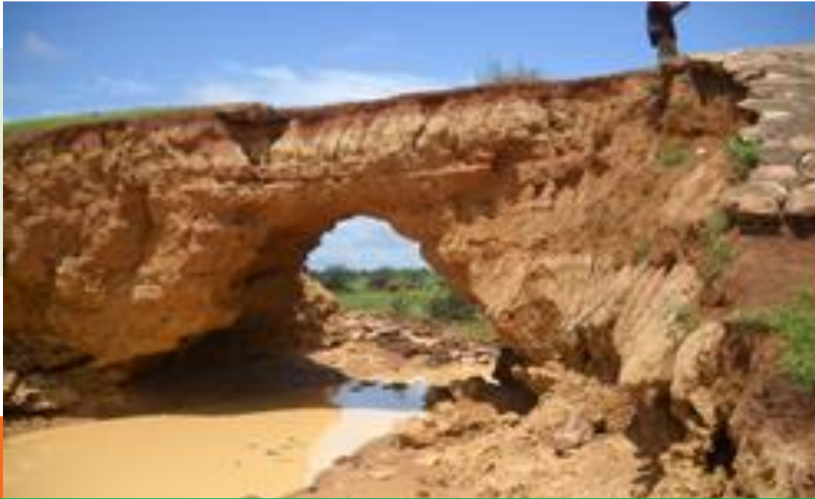
Case of internal erosion hole in a small embankment dam in Burkina Faso
