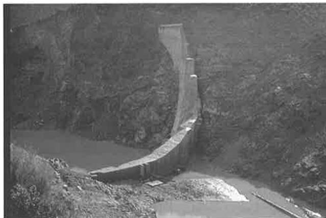
Figure 1. Remains of Malpasset arch dam: a conspicuous crevice appears along the concrete shell; the whole river discharge is flowing below the dam (photo P. Duffaut, 1960).
